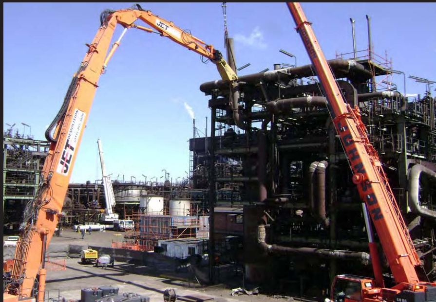
▲▲▲▲▲▲▲▲▲▲▲▲▲▲▲▲ Cold Cutting and Rigging of Petrochemical Plant in Active Process Area that Prohibits Hotwork
